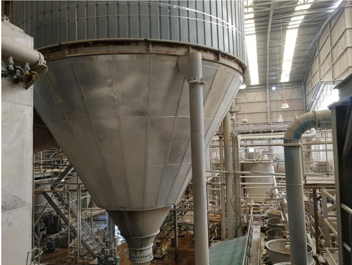
Figure 1.3 - General view of preparation unit
